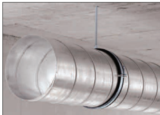
Figure 1: Circular ductwork suspended from a solid concrete slab. A knock-in expansion anchor, threaded drop-rod and noise-insulated duct ring have been used.
