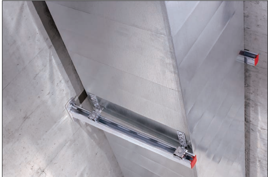
Figure 9: Rectangular ductwork in a vertical riser shaft.
