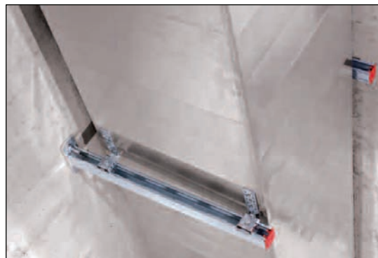
Figure 2: A ductwork riser supported from concrete riser shaft walls. Stud expansion anchors, a profiled channel system and duct angle-brackets have been used in this support configuration.
