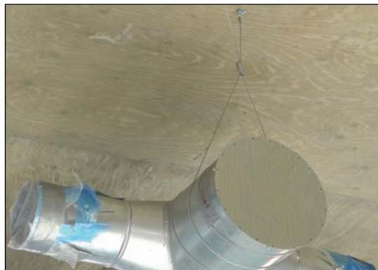
Figure 5: Circular ductwork suspended from a solid concrete slab using wire rope with a 90° end fixing. A nail anchor has been used to make the connection to the structure.
