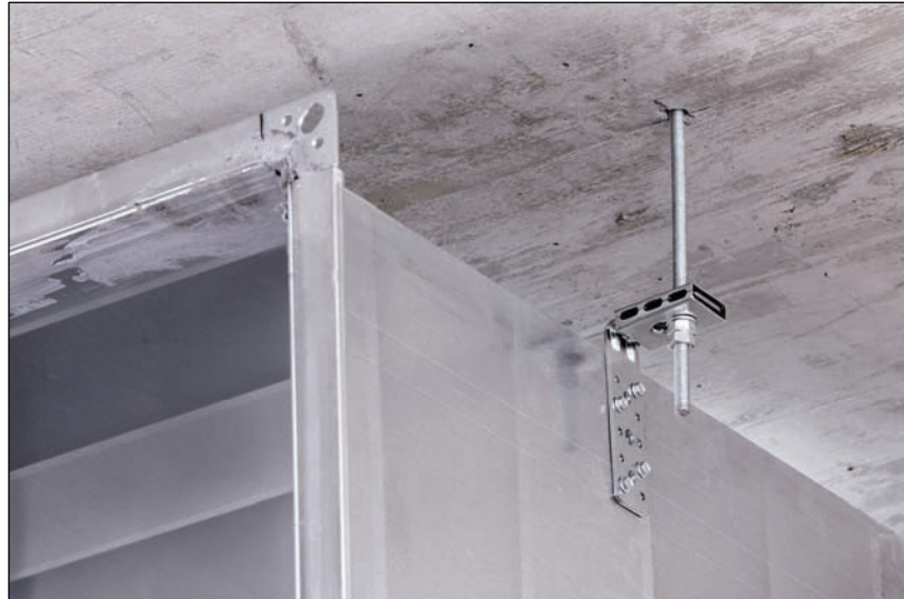
Figure 10: Rectangular ductwork suspended below a concrete slab.
